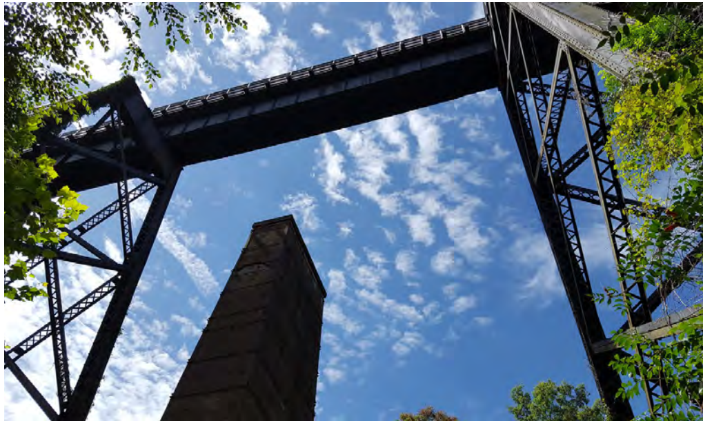
Figure 21: A steel span of the 1914 bridge soars above one of the original bridge's brick piers as viewed from below
