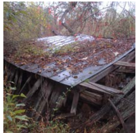
Figure 23 – Log barn at the Pratt family homestead has collapsed (2023)
